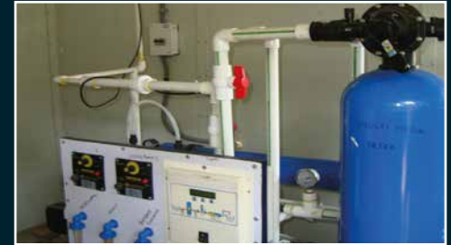
WATER FILTRATION SYSTEM
