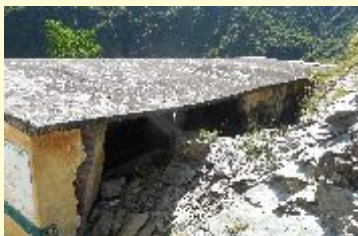
Damaged PS Mulya
